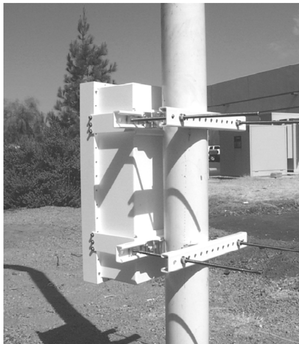
Figure C-4. Rear View of Converter Installed on Round Pole
